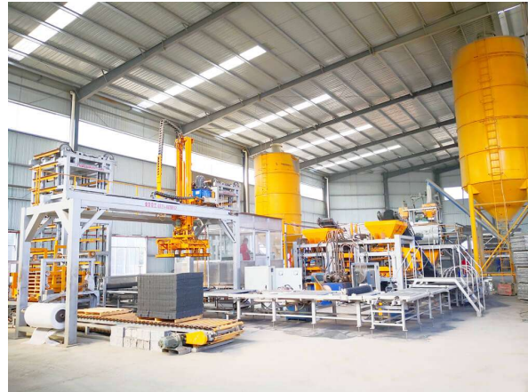
Central-control and material-handling configuration
