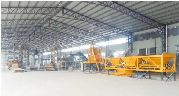
Integrated block molding and curing line
