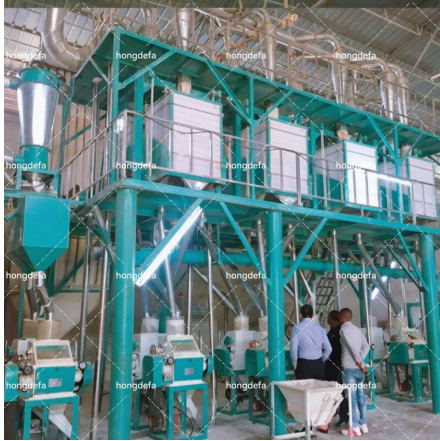
Supplier reference: installed multi-level roller-milling and sifting equipment for semolina-capable wheat processing.
